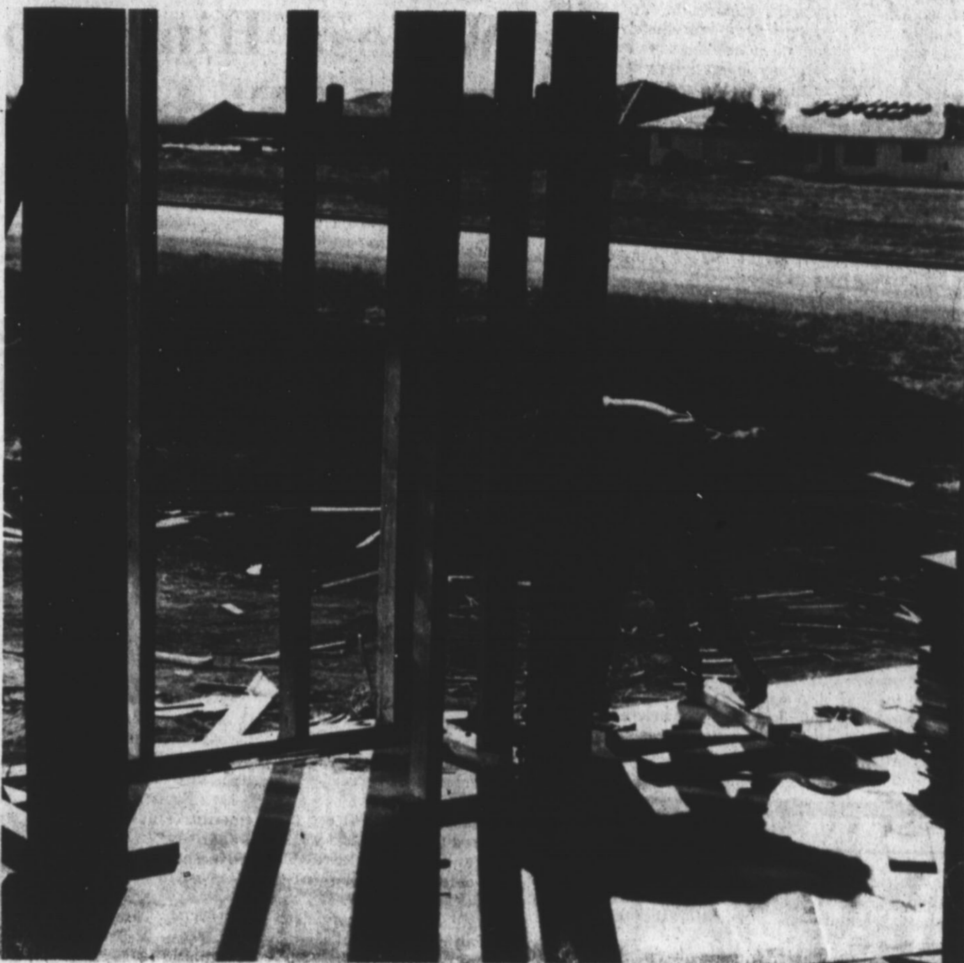
Wyatt Watkins, 341 Centre, continues work on his self-built home on Quince Street. Watkins and his wife, Frances, are doing all labor on the home themselves with the help of friends and
