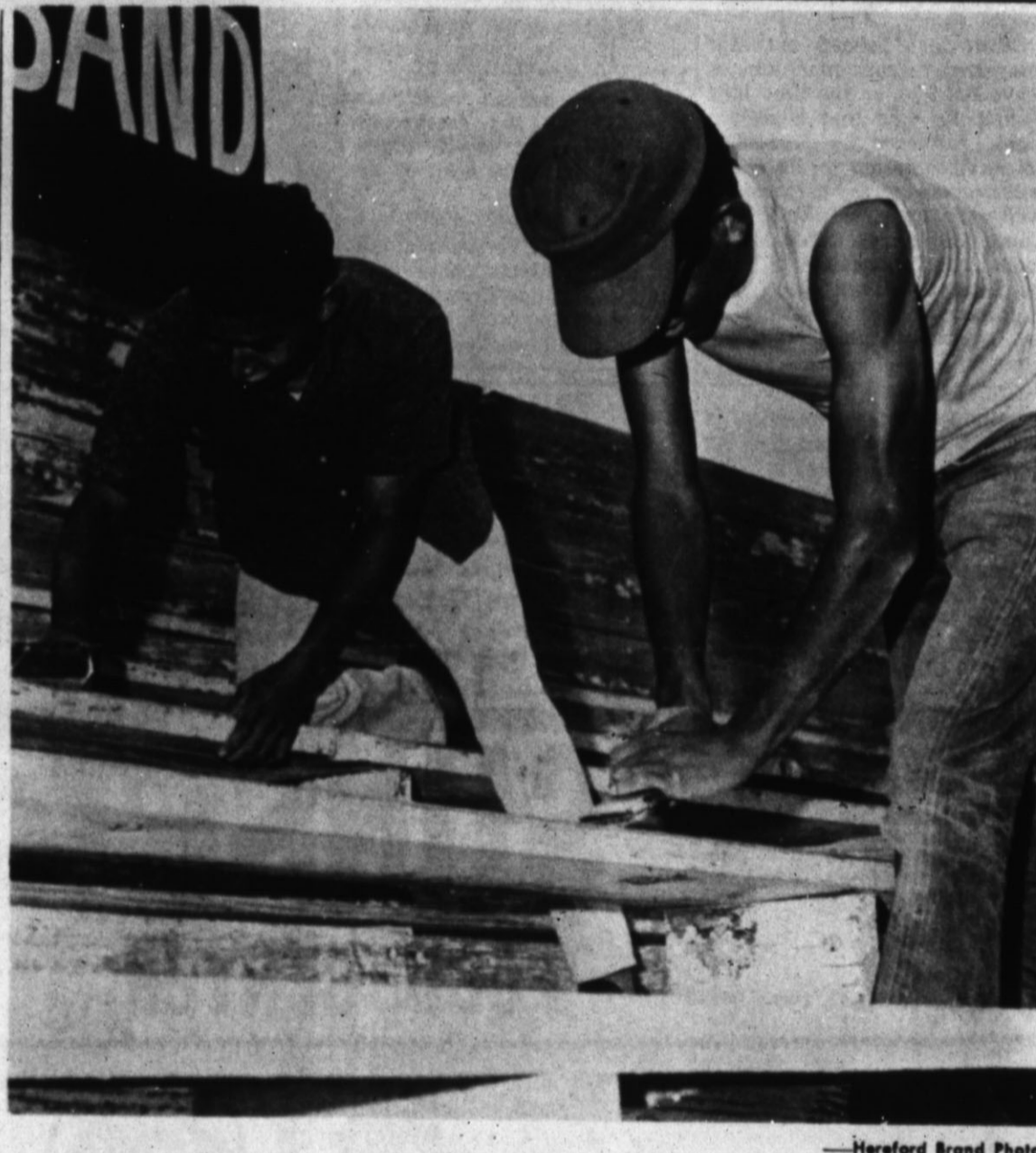
NOT MUCH LEFT TO SCRAPE — David Soto and Alfred Figueroa, employed by the Hereford schools this summer, found that there wasn't much paint left to scrape as they finished up the job at the Whiteface Stadium this week. When paint arrives, Tom Harkey, business manager at the schools, will put a contingent of Neighborhood Youth Corps workers on the project to have the stadium bright and shining in anticipation of the first football game here with Floydada Sept. 8.
