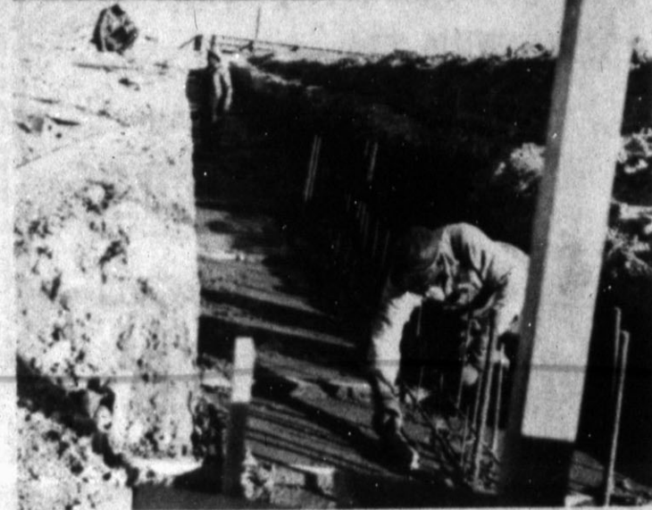
BASEMENT AND FOUNDATION — Work at the Wilson & Company beef processing plant site is just about on schedule as the foundation and other points of the large plant take shape. The top photo shows an overall view of the basement, while the bottom photo depicts some of the work being done on the building foundation topside. —Staff Photos
