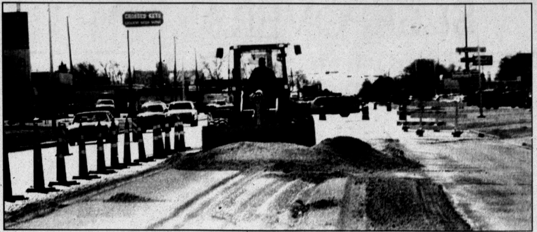
Digging up highway — A bulldozer begins to remove subsoil from the southbound lanes of U.S. 385 (North 25 Mile Avenue) near the Northgate Plaza shopping center. The work is part of
