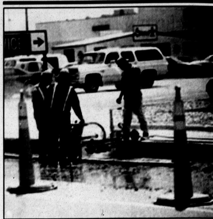
Getting ready to pour — Construction workers prepare the roadbed in the 500 block of North 25 Mile Avenue for pouring of concrete. Asphalt has been sprayed and workers smooth the sides of the roadway in preparation for the pouring of concrete.
