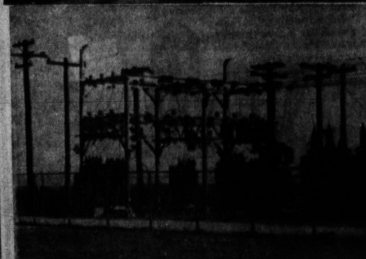
THE NEW REA SUB-STATION, above, is entered on the record as No. 9, and will split the electric load for the west part of the county. It has 5,000 KVA capacity and, when put into operation this week, was serving 300 customers, including 50 irrigation wells. The capacity will handle up to 150 irrigation
