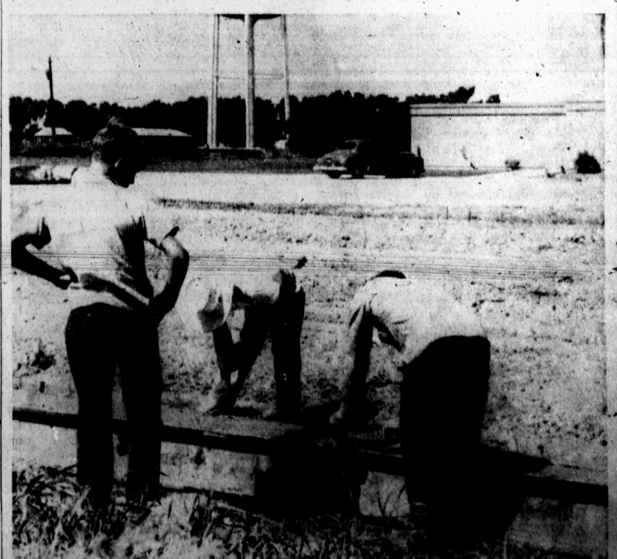
PAVING FOR MOREMAN STREET is within two weeks of reality as Parker Brothers Construction Co. of Hereford started grade work and pouring curb and gutter around Northwest Elementary School and east to U. S. Highway 385. Work started Monday and should be completed within two weeks.
