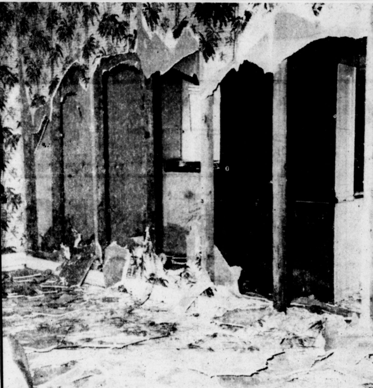
VANDALISM DAMAGE to a vacant house at 122 Moreman St. last week amounted to nearly $300. Five Hereford youngsters, ranging in age from six to 10 years, were accompanied by their parents in a juvenile
