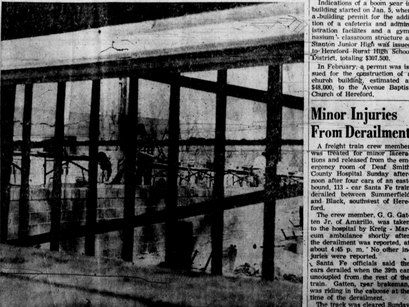
ONE OF MANY construction projects in Hereford started in 1959 is the new county jail. Framed by newly-installed window bars, brick layers erect the walls for the structure. Bad weather and material delays have hampered speed on the project, but the construction supervisor says new work is about on schedule. The building is to be completed about Aug. 1. (Staff Photo)
