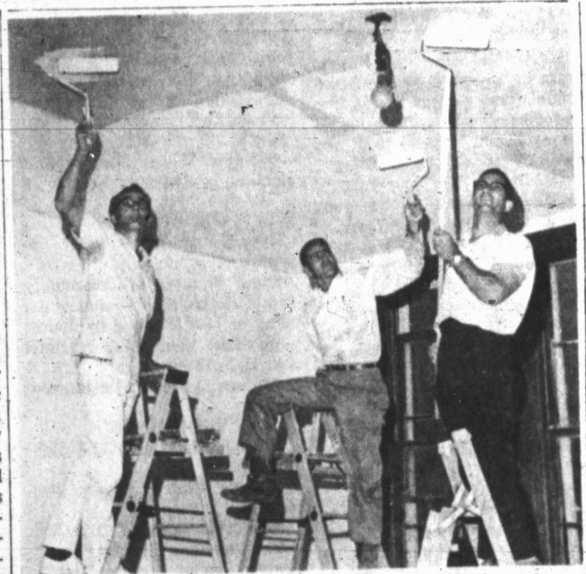
PAINTERS WITH A PURPOSE — Hereford Jaycees members Troy Vinson, Dick Kendrick, and Wayne Houlette, from the left, are among members of the Jaycees who have donated services to remodel the interior of the Deaf Smith County Museum building. (Staff Photo)
