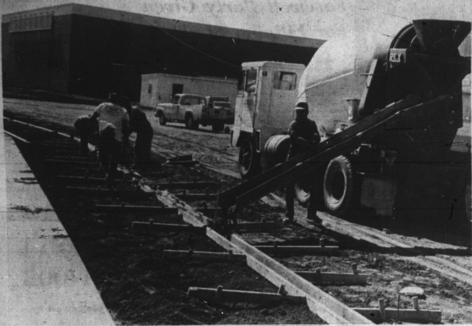
LADDER EFFECT — Sidewalks at LaPlata Junior High were being poured this week as construction went into last phases on the new structure. (Staff Photo)
