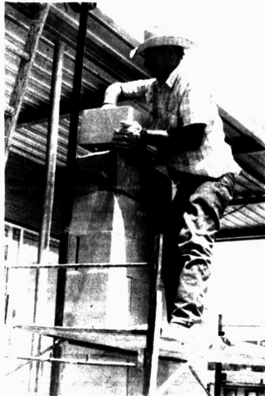
Jerry Hix of Hereford adds another cinder block to the stack for the remodeling project going on at Panhandle Community Services, 603 E. Park in Hereford.
