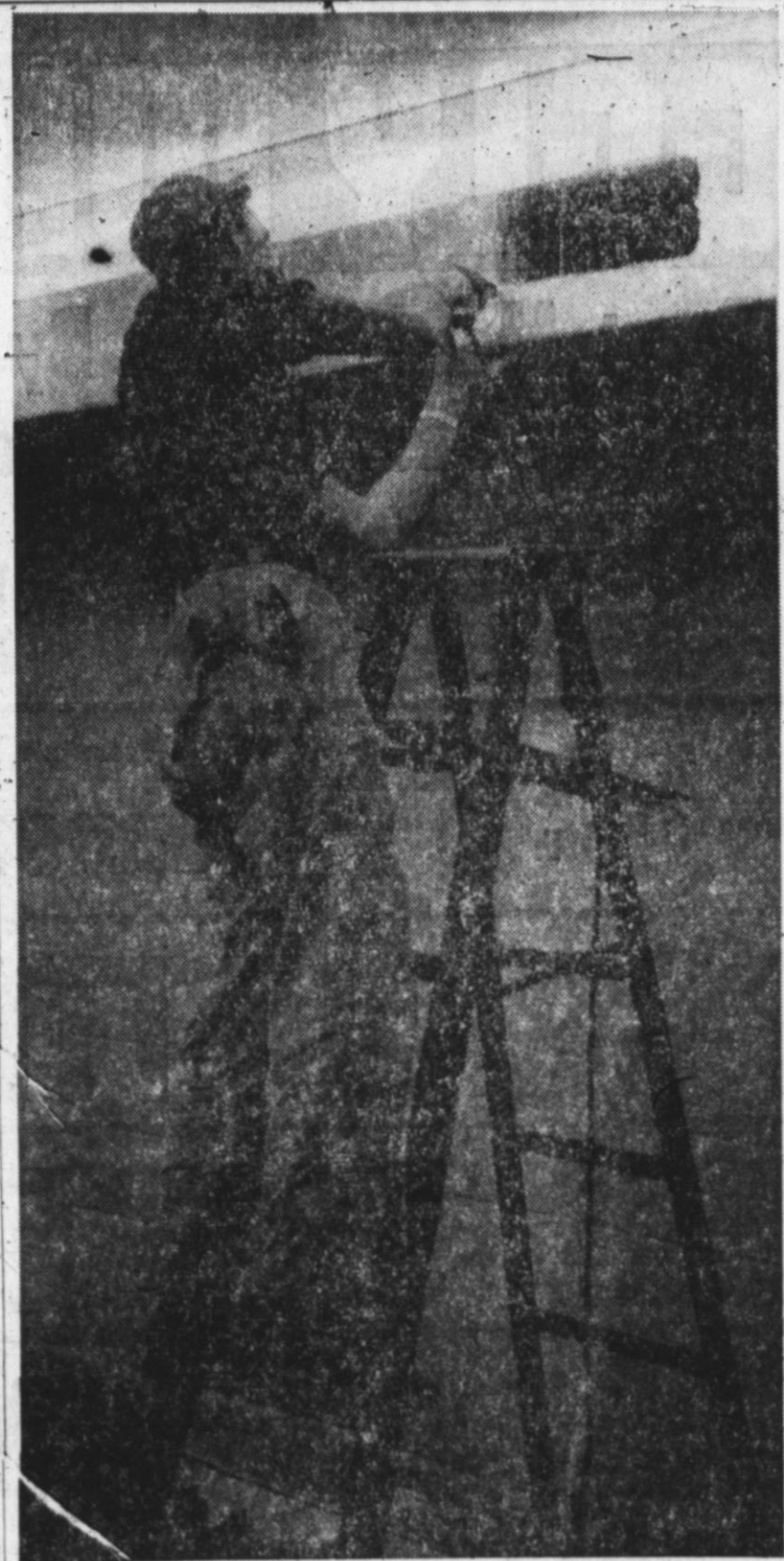
WORK IS progressing on medical research laboratory at Fourth and Miles. John Hix of Brown Sheet Metal Co. is shown installing wiring for air conditioning Tuesday. Installation of laboratory equipment is to start today. The lab is supposed to open May 17. (Staff Photo)
