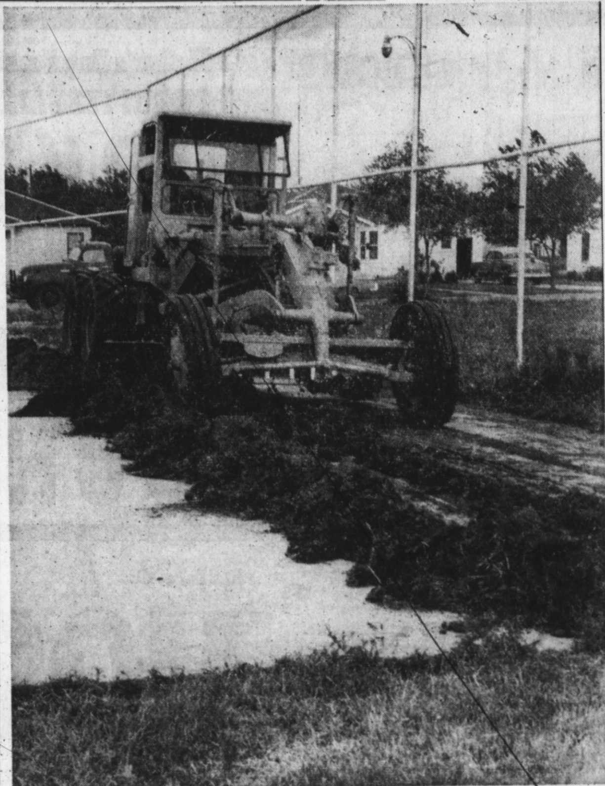
IMPROVEMENTS ON COURTS—City workers began Tuesday afternoon clearing earth for the pouring of concrete around the tennis courts, which is to be completed in time for the Invitational Tournament Friday and Saturday. Concrete will be laid between the courts and back screens, and also between the two courts. Grass will be left on the outside of the courts. (Staff Photo)
