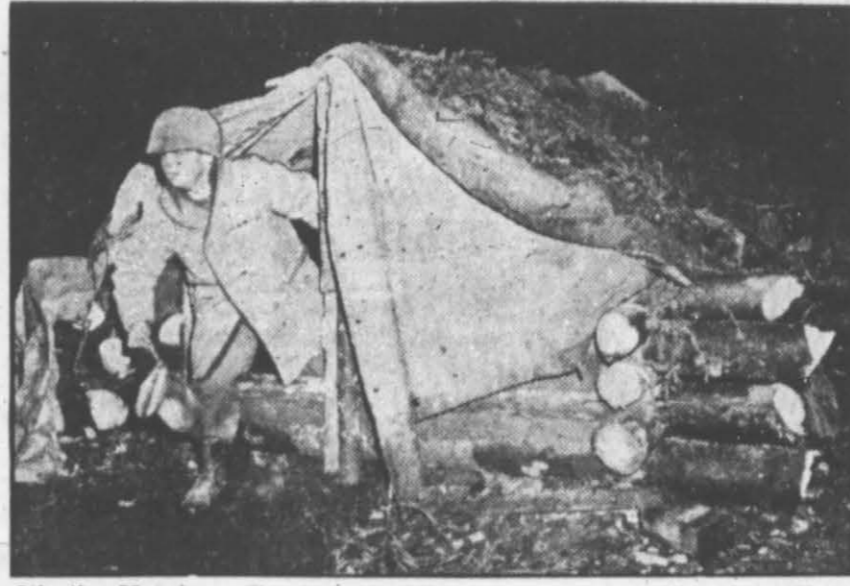
It's the Huertgen Forest-style Nissen hut. American soldiers are building them for protection against snow and cold in Germany; chunks of clay, tarpaulin roof, brown paper from cement bags for wall insulation is standard construction. That's Pvt. Theron McCravay of Chester, S. C., who has just heard chow call.
