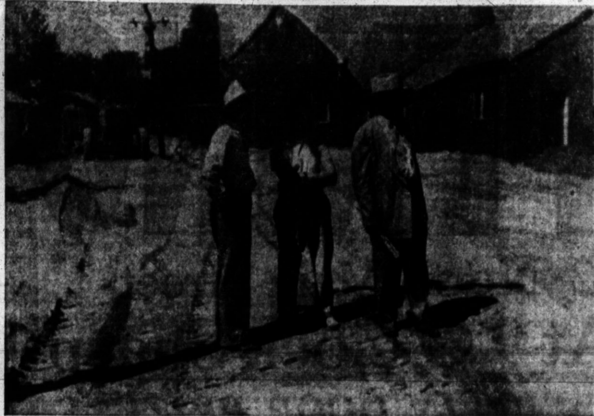
STUDYING THE SITUATION —Rev. Don Davidson, right, Bruce Miller and Hugh Clearman look over the partly completed new Methodist parking lot behind the church.
