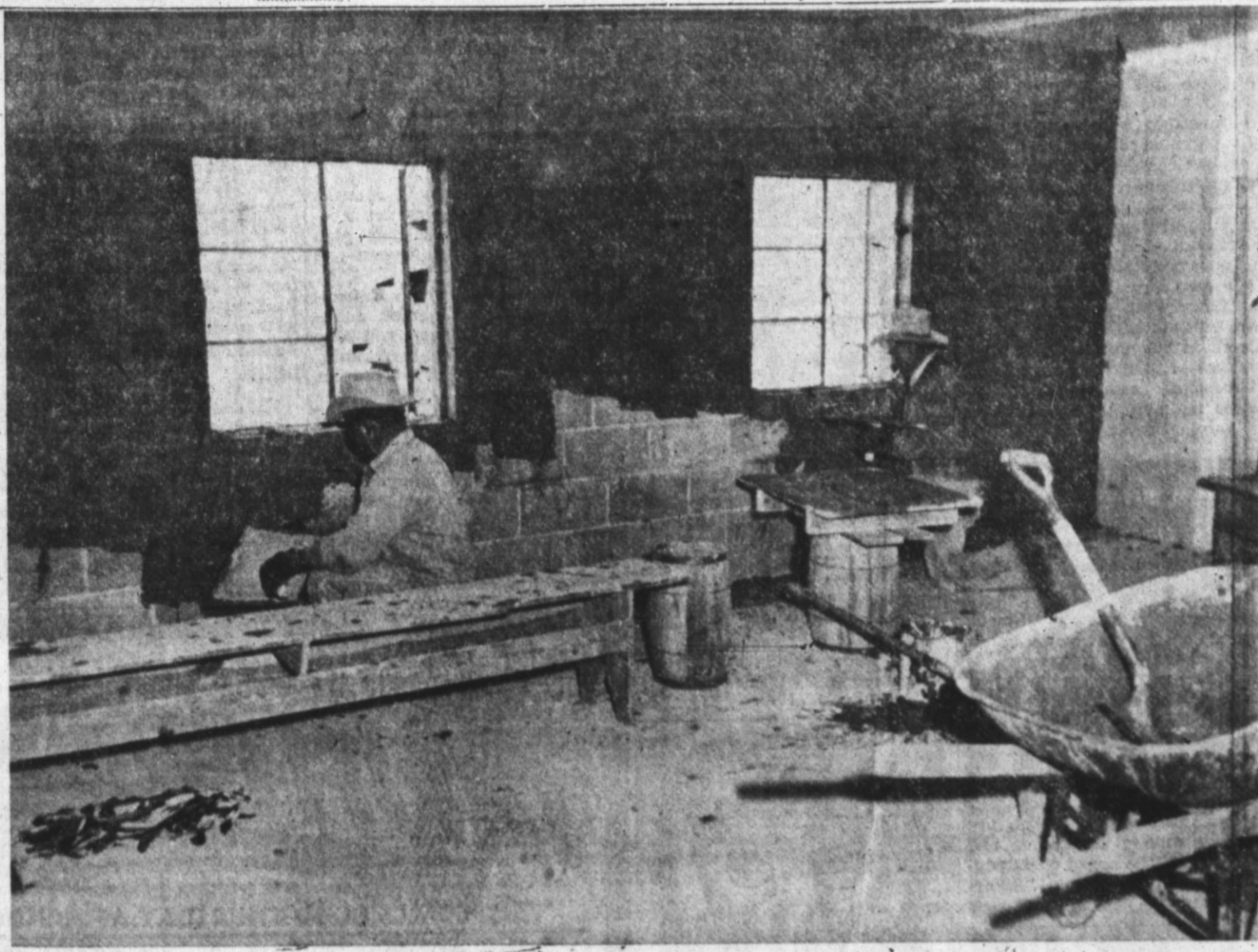
IT WON'T BE LONG now before the new hospital for the Mexican Labor camp is ready for use of residents of the camp. The hospital was built mostly by Father Raymond Gil-
