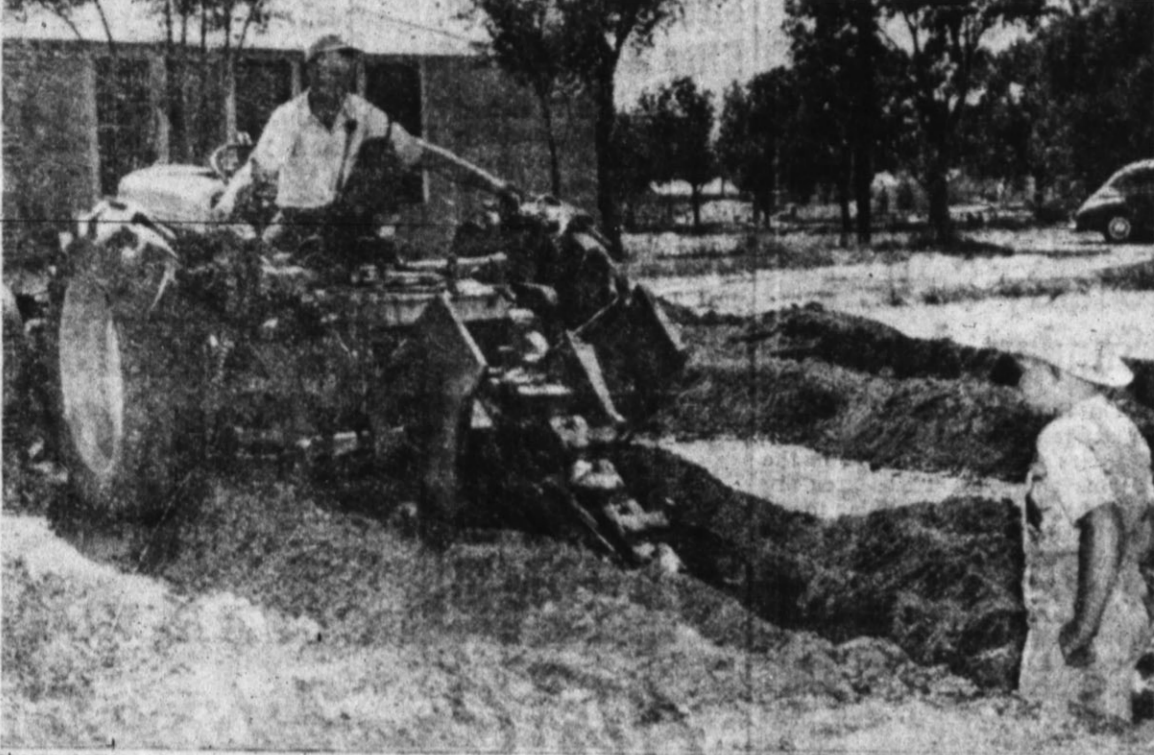
WORKMEN ARE BUSY in Friona digging up old water pipe and relaying new across streets to be paved in the town's current paving program. Leslie Weis, above, is shown operating a trenching machine to lay new pipe across the street. His brother, Bobby Gene Weis, is watching the work. —Brand Staff Photo
