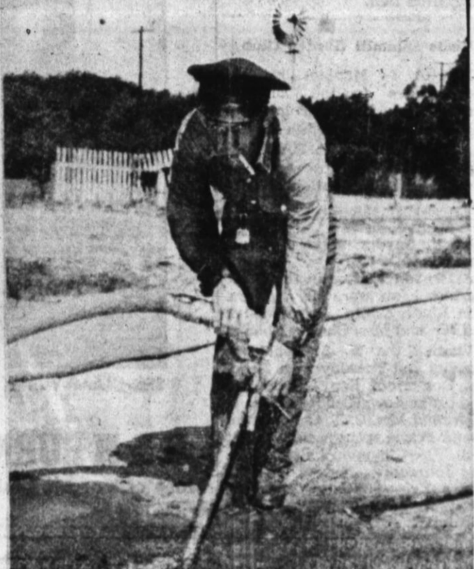
ROBERT HOLLIS is shown sinking the ground around the old water pipe on Friona's streets before they are taken up. Hollis is a city employee. Construction work on the pavement is being done by Brown and Root. —Brand Staff Photo
