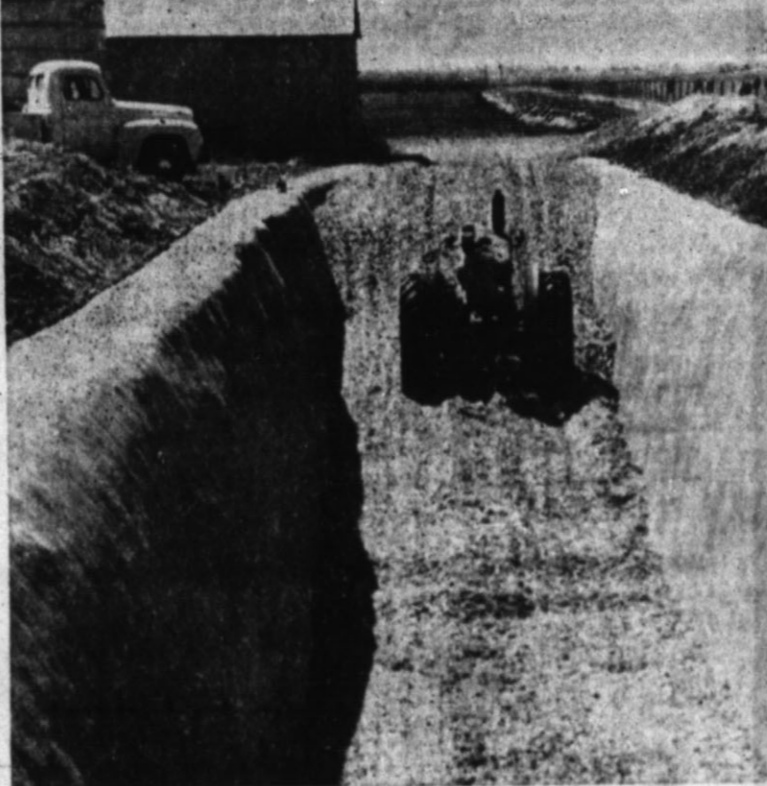
Evans got his idea of plastering the walls of the silo from T. E. Baldrige, who operates similar silos at Portales. Experience has a saving in wall cave-ins and cleaning, putting the silo on a more permanent basis.
