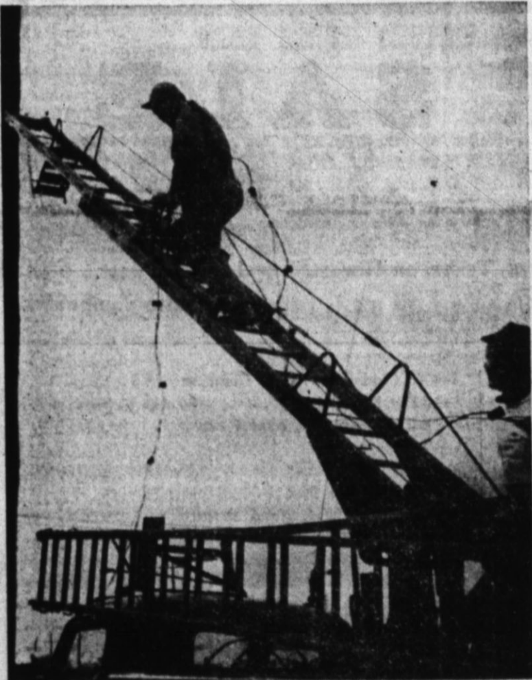
NOT LACKING FOR the proper equipment to do their job, Jaycees climb up a pole with the aid of a Southwestern Public Service truck. High man on the ladder is Dub Reeves. At lower right is Otis Hall.
