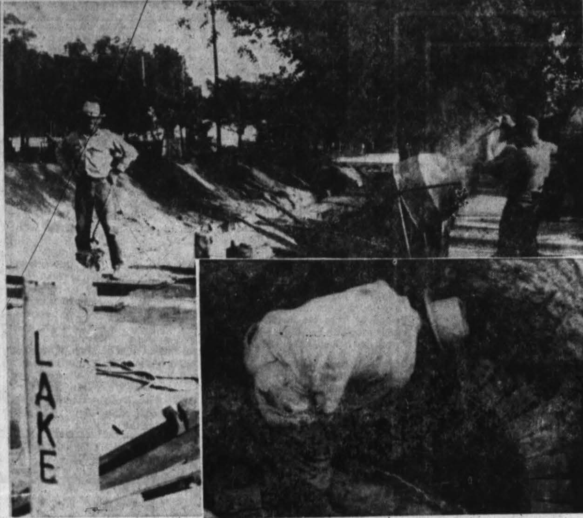
WORK ON 25 MILE AVENUE -- You can call C. W. Gresham, left, and Carl Stafford the upper men and Arthur Stafford, pictured in inset, the lower man in this operation. Gresham and Carl Stafford are busy on top of the ground preparing and lowering cement and bricks to Arthur Stafford, who is in the hole Gresham is standing over. Actually the hole is a lot deeper than it looks and is far over Stafford's head. (Staff Photos)
