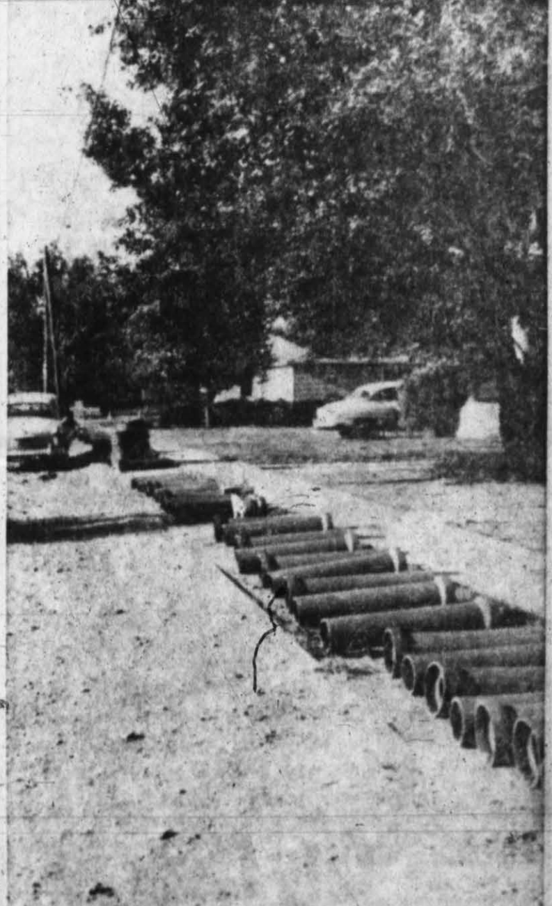
FIRST ACTUAL WORK -- First visible work on the Highway 51 widening program got underway last week when workmen began preparing to lay the new sewer line. Pictured here is some of the pipe placed along 25 Mile Avenue which will be used in the project. (Staff Photo)
