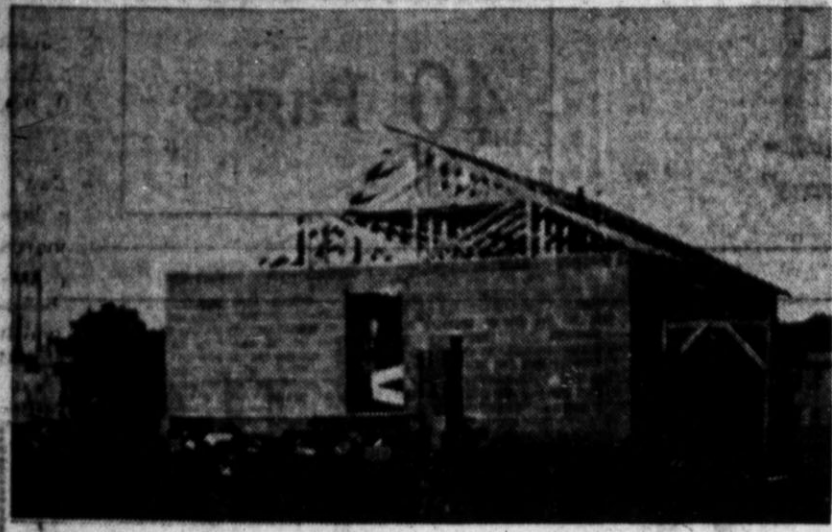
WORK ON THE SCHOOL for Negro children in Hereford has progressed quite rapidly, as can be noted from this picture taken Friday afternoon. The building is supposed to be ready when school opens for all other children Tuesday morning. (Staff Photo.)
