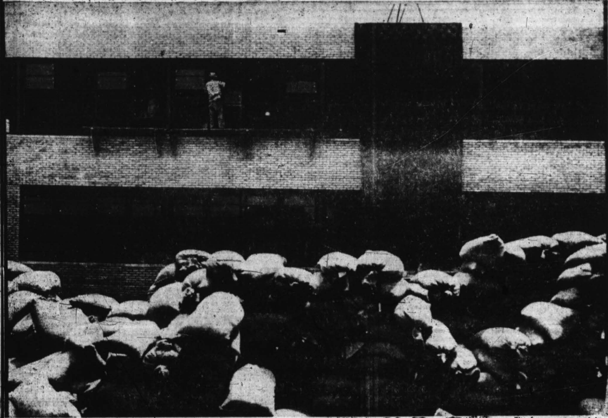
WINDOWS ARE AMONG the very last things to go into the outside of a new building these days, and their installation means that most of the outside work is finished, even though there is still much to be done on the inside. In this case, steel casements were being put up on the West side of the new
