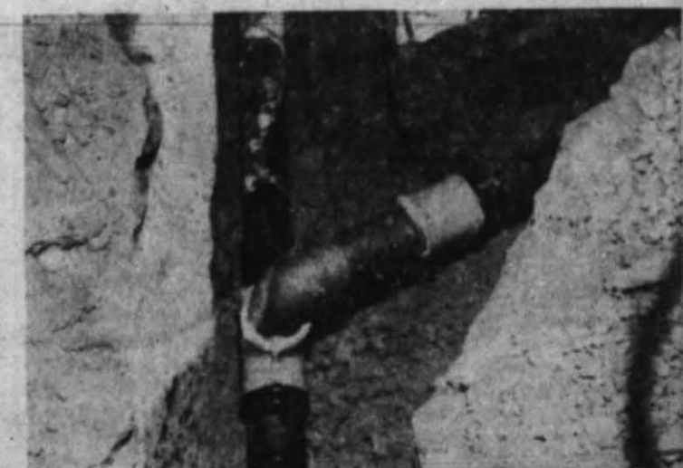
Miles and miles of CARLON GAS PIPE are all ready in service on the High Plains. A list of satisfied users is available on request.
