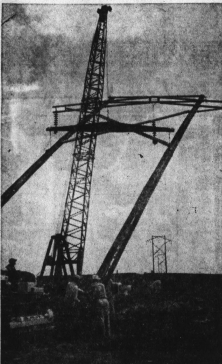
SAFETY MEASURE—For greater safety in erecting the massive 75 foot structures they were "put together" on the ground and raised into position with a 60 foot crane on an Athey Wagon. These structures will stand the pressure of a 160 mile an hour wind.
