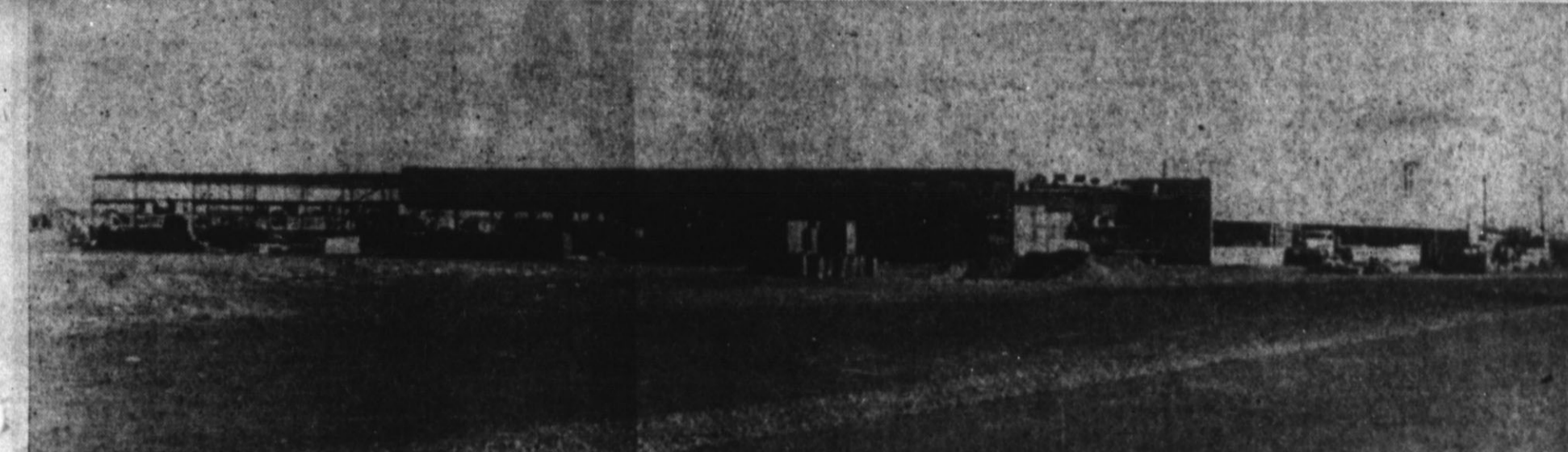
SCHOOL TAKES SHAPE—The new Ela Aikman Elementary School has started to take on a new look in the last few weeks, as workmen rush to get the school completed in time to be used during the next term. It remains the largest building project in Hereford at the present time. (Staff Photo)
