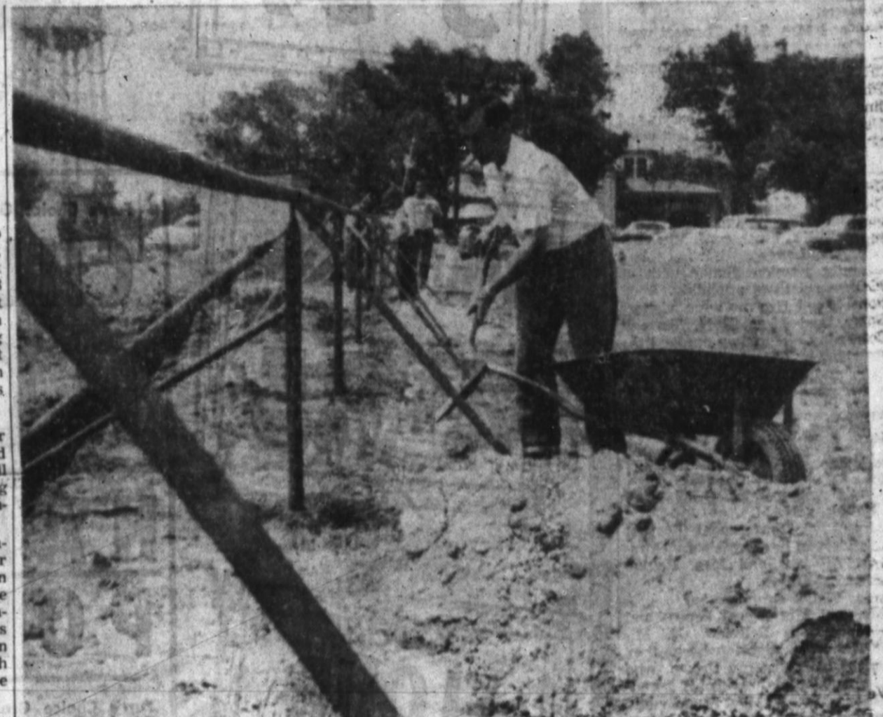
POURING CONCRETE—Jimmie Bounds pours concrete around a post down the left field line. The fence will be of pine framework and chain link fence. The outfield fence will be metal. (Staff Photo)
