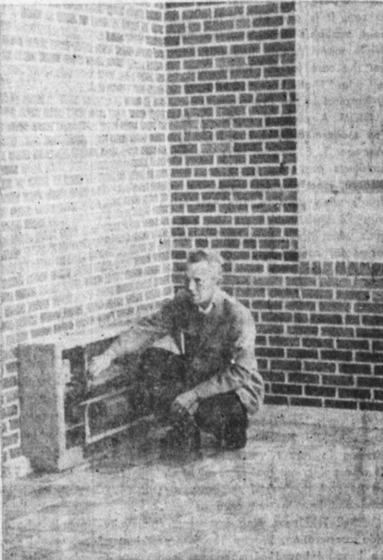
CHECKS AIR CONDITIONING INSTALLATION—Paul Coneway, Hereford district manager for Clowe & Cowan, Inc., is shown in the solarium at the new Children's Wing of the county hospital, giving one of the air conditioning units a final check as installation neared completion. Coneway's firm presented the $5,900 heating and air conditioning unit in the hospital addition as a gift from the customers of Clowe and Cowan. (Staff Photo)
