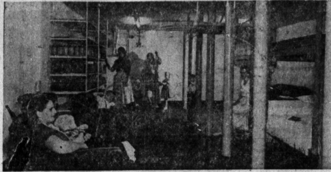
THE ULTIMATE in family shelters is represented by this large and luxurious unit built by steel contractor Earl W. Reichert of Battle Creek, Michigan. The $10,000 structure has a 98-foot well, private electric generating plant, electric and hand-operated blowers for the filtered air system. Its steel reinforcement prepares it for use as a blast as well as fallout shelter. However, a small family fallout shelter may be built for a fraction of what this shelter cost. (Battle Creek Enquirer and News Photo)
