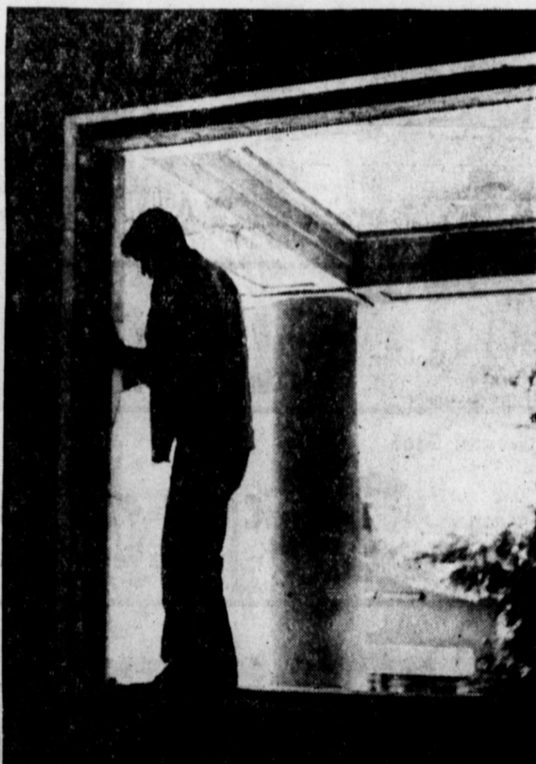
WITH NO CONCERN, this worker readies an opening for new aluminum windows in the district courtroom. He's working three stories up, but doesn't let that distract him . . . much.
