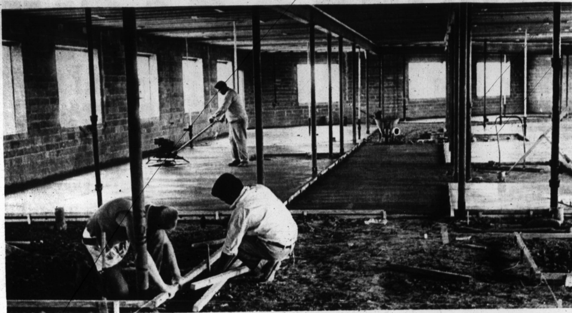
INTERIOR WORK AT KING'S Manor was progressing this week as workmen began setting the forms for concrete floors, electrical outlets, and pouring the floor. Floors in the east wing of the building have been completed and construction shifted to the west wing. The first unit of the home for the aged is expected to be completed in the fall of the year and ready for occupancy. Cost of the unit is $166,103. (Staff Photo)
