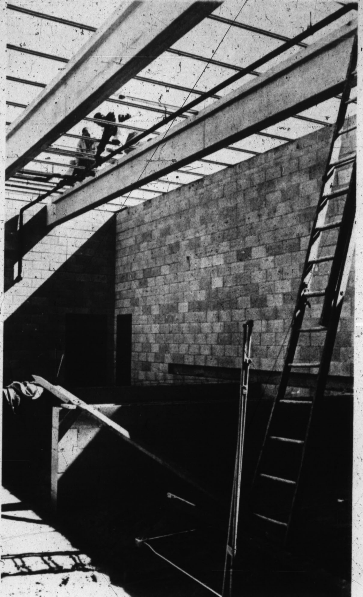
AT NORTHWEST ELEMENTARY SCHOOL workmen install ceiling pipes before the roof and ceiling of the building are constructed. The building will provide additional classroom space and office space plus a cafeteria. Work on the expansion project began here in November and is expected to be completed by the time school opens in the fall of 1963. (Staff Photo)
