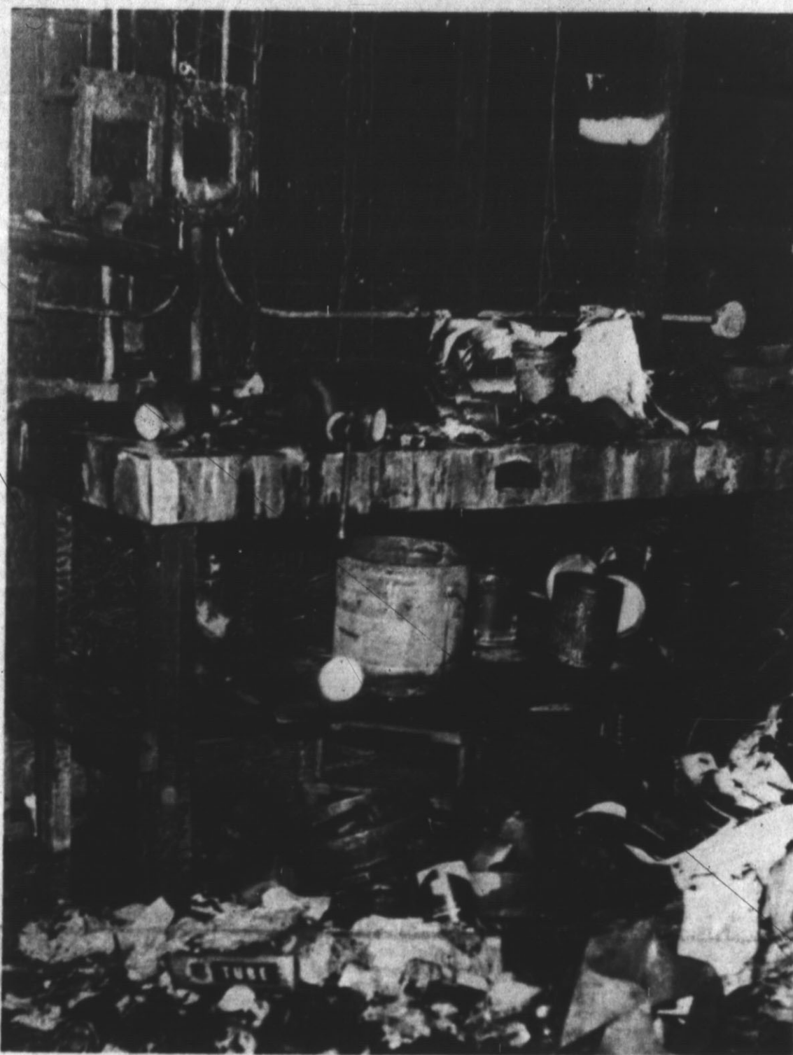
A FIRE STARTING IN this store room is an hour after the station closed. Volunteer firemen battled heavy smoke from burning tires and oil in order to extinguish the blaze. The blaze was reported about 10:35 p.m. (Staff Photo)
