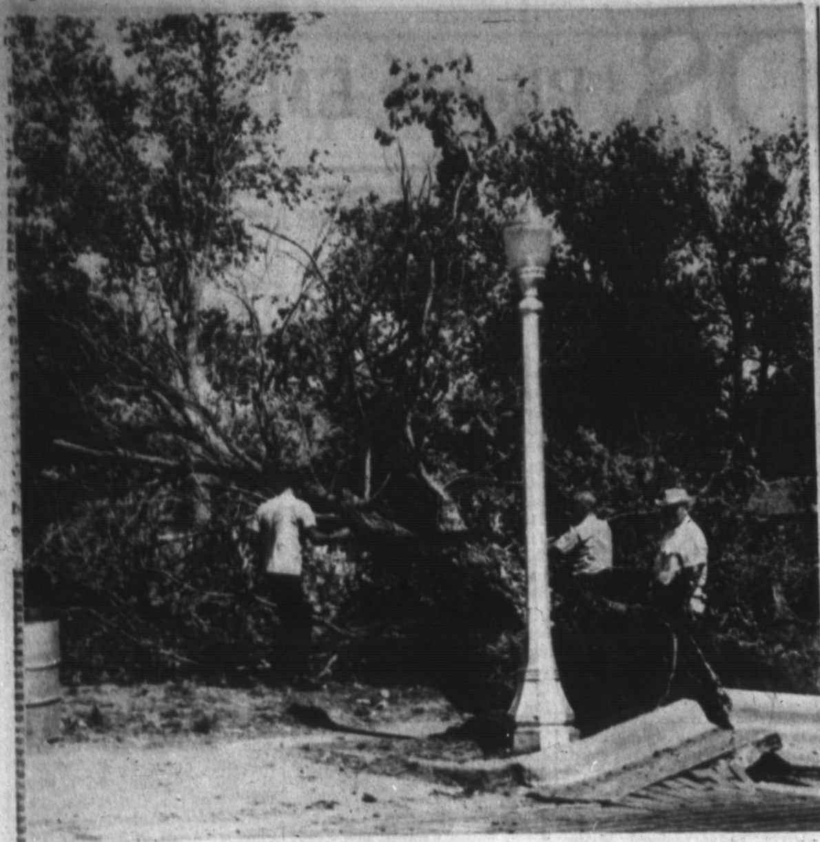
CLEARING OFF TREES — Workers are shown here clearing off trees on the lot belonging to Deaf Smith County, north of the court-
