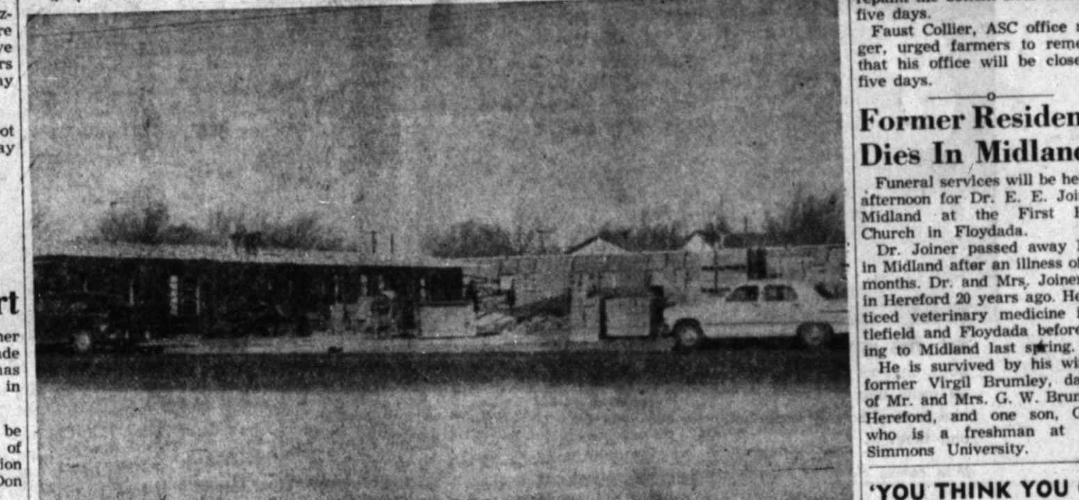
GOING UP FAST — Probably the fastest rising buildings in town are the ones pictured above. They are the site for the M. S. Benefield motel. The motel is modeled after one in California, and is expected to be one of the Panhandle's most modern. (Staff Photo)
