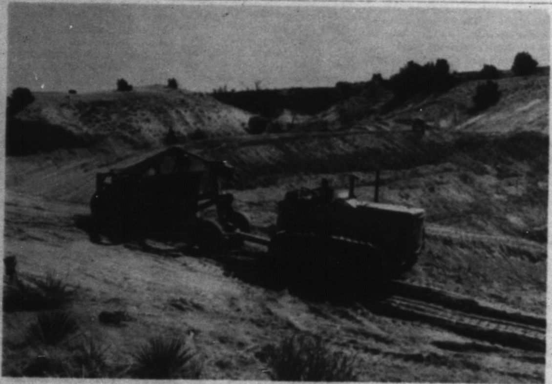
RONALD MATTHEWS, a 25-year employee of the Soil Conservation Service is shown above operating some of the heavy equipment needed in building farm ponds. (SCD Photo)
