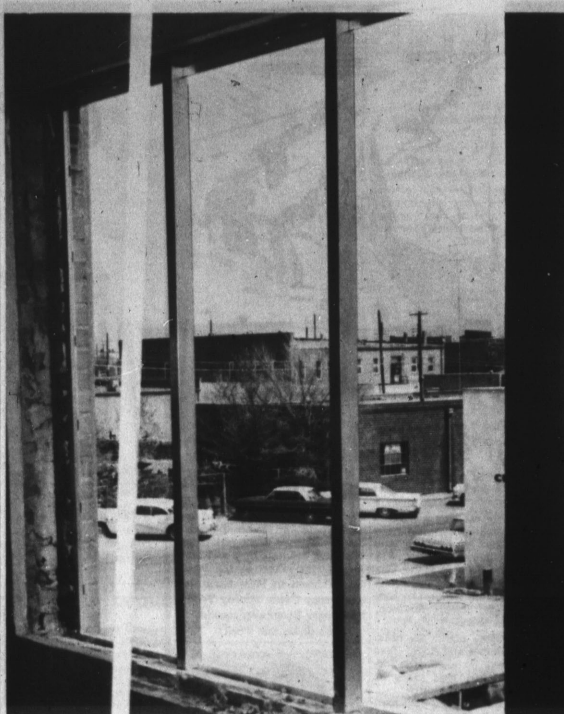
NEW WINDOWS — New windows being installed on the second floor of the city hall went up rapidly this week. This window is in the chief of police's office. The new windows will allow the building to be centrally heated and air conditioned at less expense. (Brand Staff Photo)
