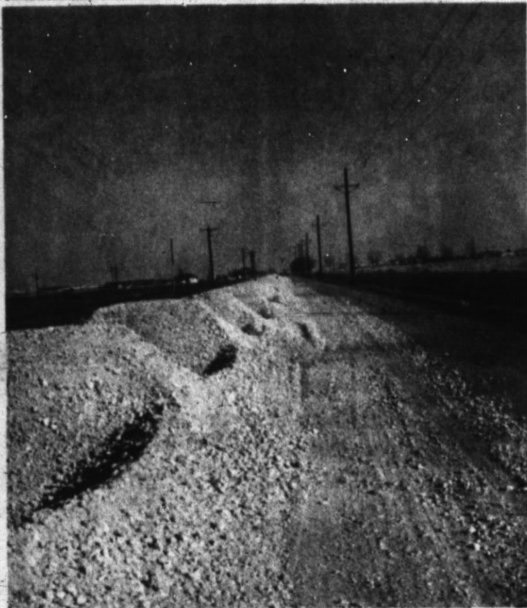
SIGNS OF PROGRESS — Caliche base is being spread on the part of Fifteenth west of Highway 385. Paving on that portion of the street, being done by the county, will make access to LaPlata Junior High more convenient.
