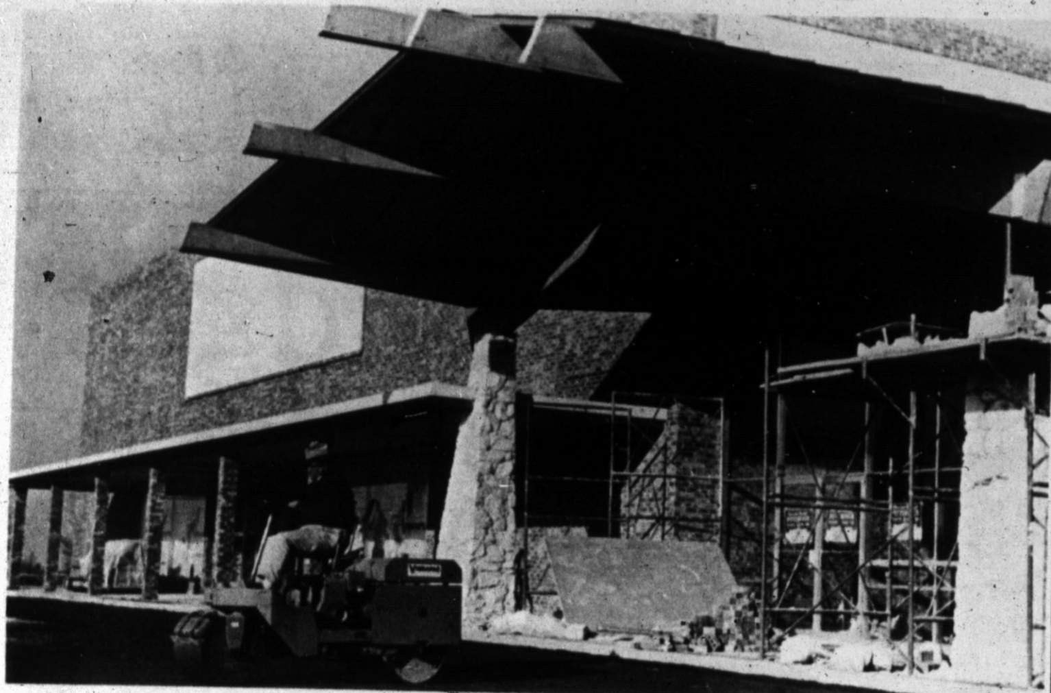
OUTSIDE WORK PUSHED — Exterior work at Sugarland Mall Shopping Center is nearing completion, as several stores are planning a March 2 opening in the north Here-
