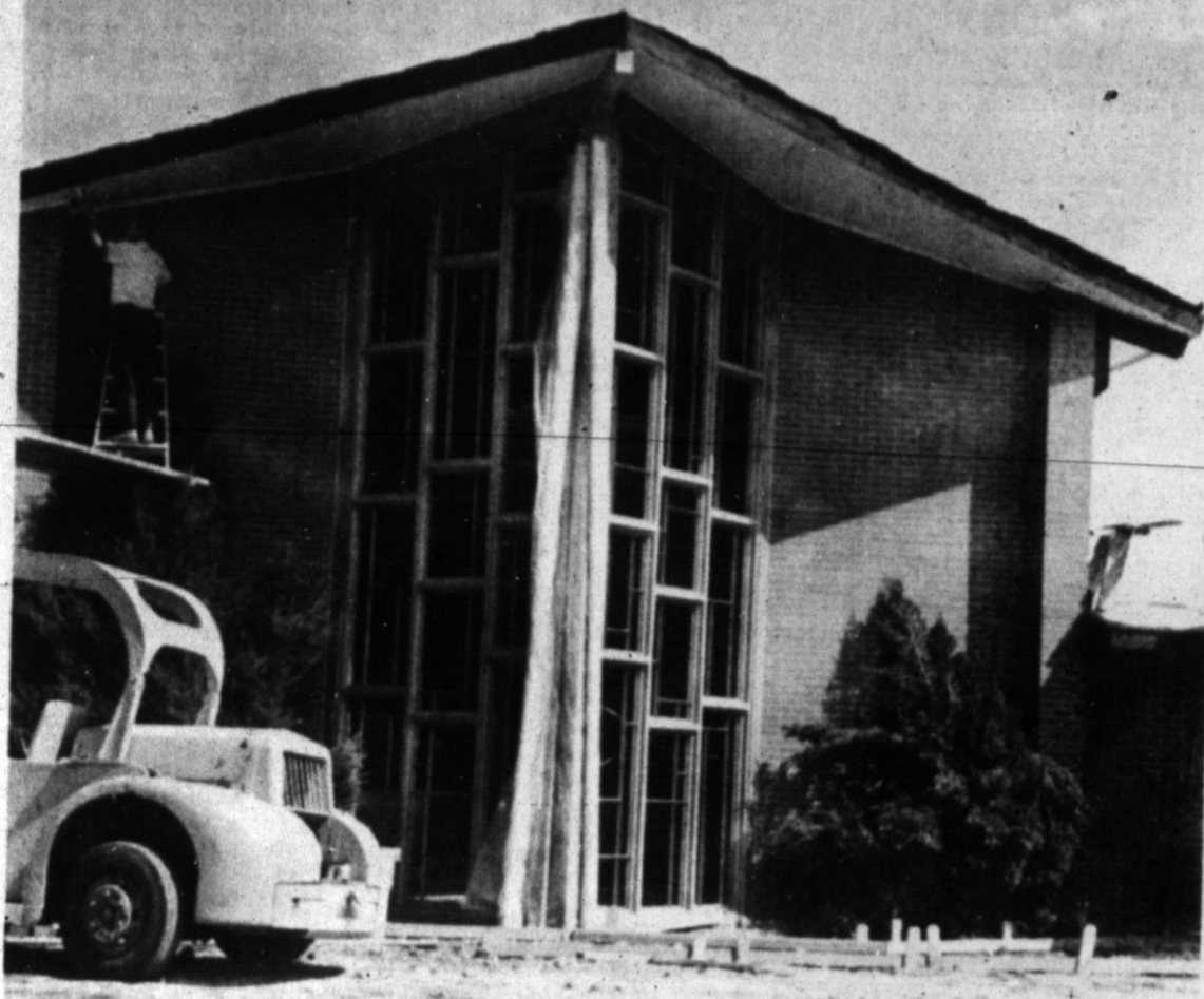
SIGNS OF PROGRESS — Removal of a neon cross framing entranceway at St. Thomas Episcopal Church on Harrison Highway has changed the looks of the building. Stained glass will be placed in the ceiling-to-floor frame now installed. Construction is nearing completion on the remodeling and expansion program at the church. (Staff Photo)
