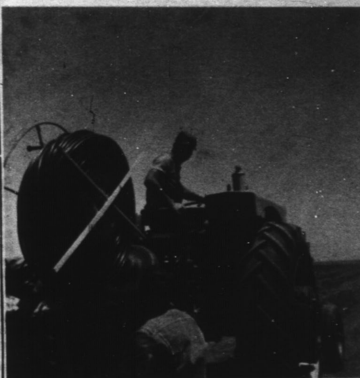
PIPE PLANTING OPERATION — G. V. Hall, left, and Keith Henderson adjust the pipe planting machine during laying of the underground pipeline, as Elmo Hall watches from the tractor seat.
