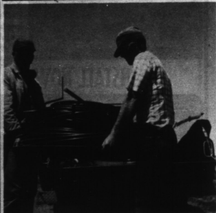
IRRIGATION LINE ARRIVES — The Hall brothers, Elmo at left and G. V., are shown unloading the plastic underground irrigation pipe just prior to putting it in the ground.
