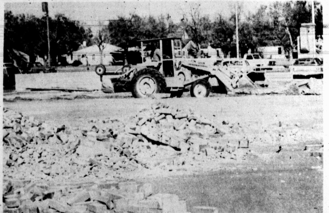
WORK BEGINS —Construction on the $190,000 First National Bank addition started recently as workers began tearing down buildings on the
