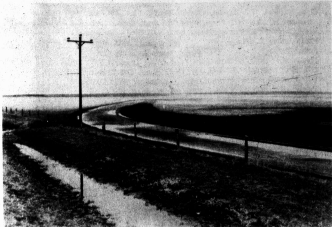
DIVERSION TERRACE — This diversion terrace, constructed through the Great Plains Conservation program, helped divert water from a county bar ditch onto empty range-
