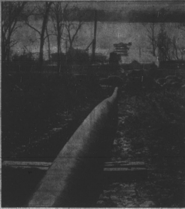
A part of the Magnolia Pipe Line Company's 650-mile, 20-inch crude oil line, extending from Corsicana, Texas to Patoka, Ill., may be seen at the Mississippi river crossing near Chester, Ill. This is the largest big-inch crude oil pipe line constructed since the war and will pump 100,000 barrels of oil a day. In the river can be seen the derrick barge, ramp barge and pontoon boats that took part in the river crossing operations.—(AP Photo).
