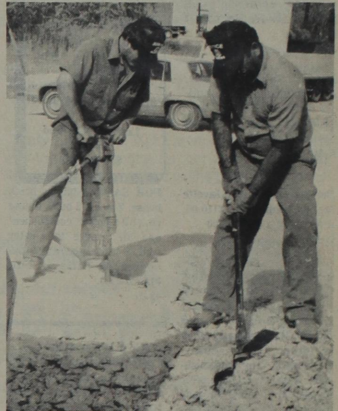
James Horrell uses a grubbing hoe and Billy Justice uses a jackhammer to reduce the cracked and worn sidewalk in front of the Rising Star Post Office to rubble. A new sidewalk is just one of the renovations in store for the post office.
