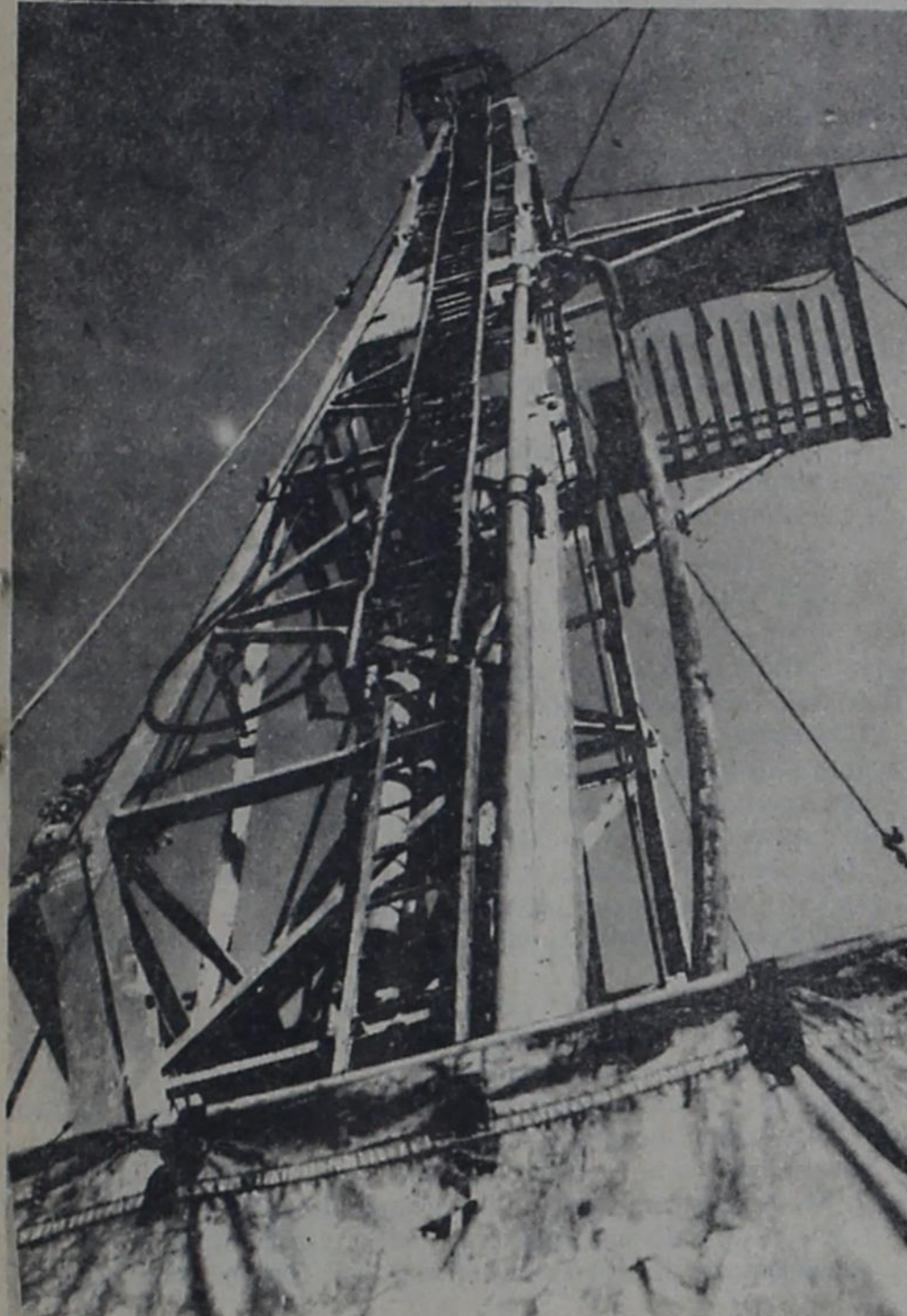
Looking up the rig of a new well on the Massman lease on the Clarence Stroebel ranch.
