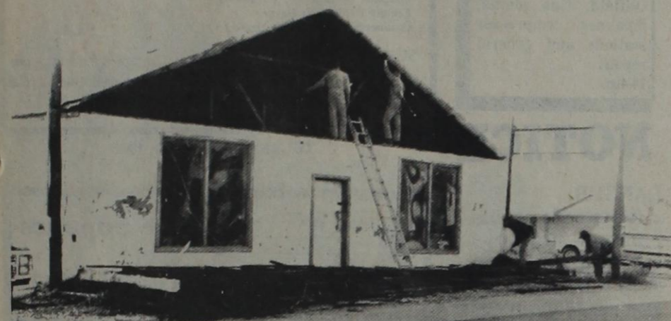
Destructive winds collapsed the false front of the building on N. Main occupied by P.M. Water Well Service. David Pollock and Charlie Moore, who operate the business, didn't see any humor in Mother Nature's April Fool's joke as they began cleaning up the mess she made.
