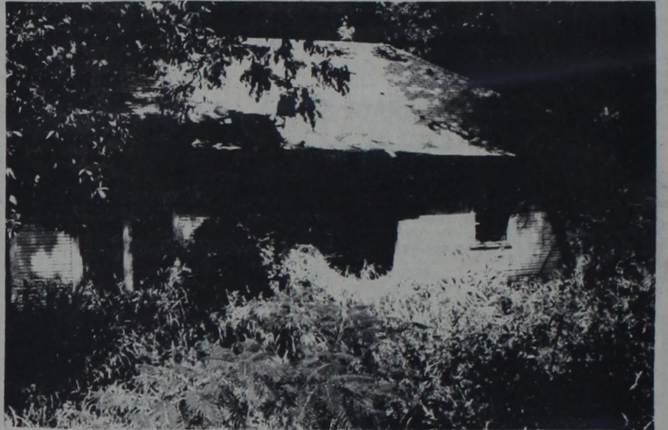
Fire severely damaged this house last week. The George Stone family lived here. Watch for a story in the next issue.
