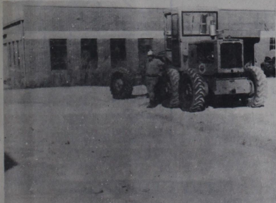
Duby Jones puts the finishing touches on spreading the caliche around the post office.
