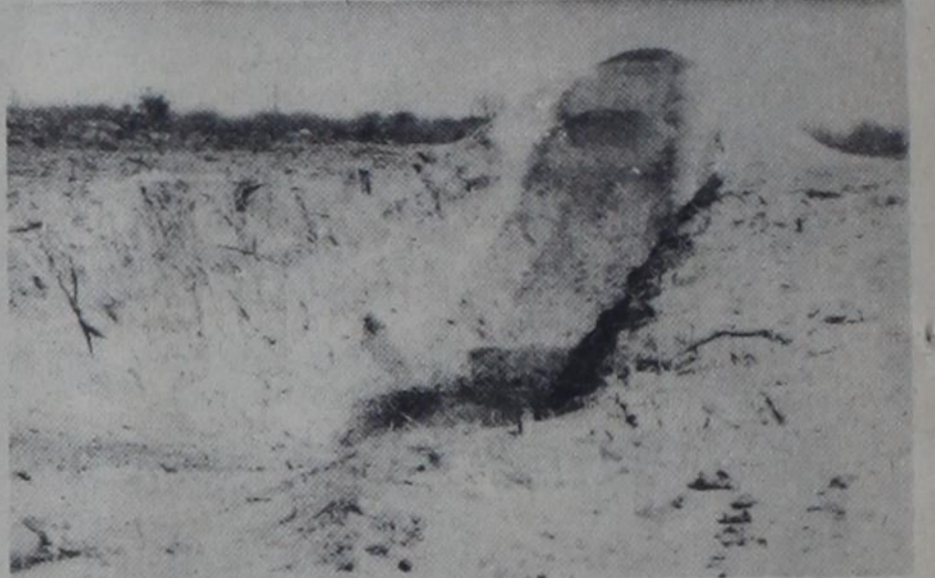
Future sight of the sanitary landfill located two miles northeast of the city just off cemetery road. Shown above is the test pit dug some weeks ago.
