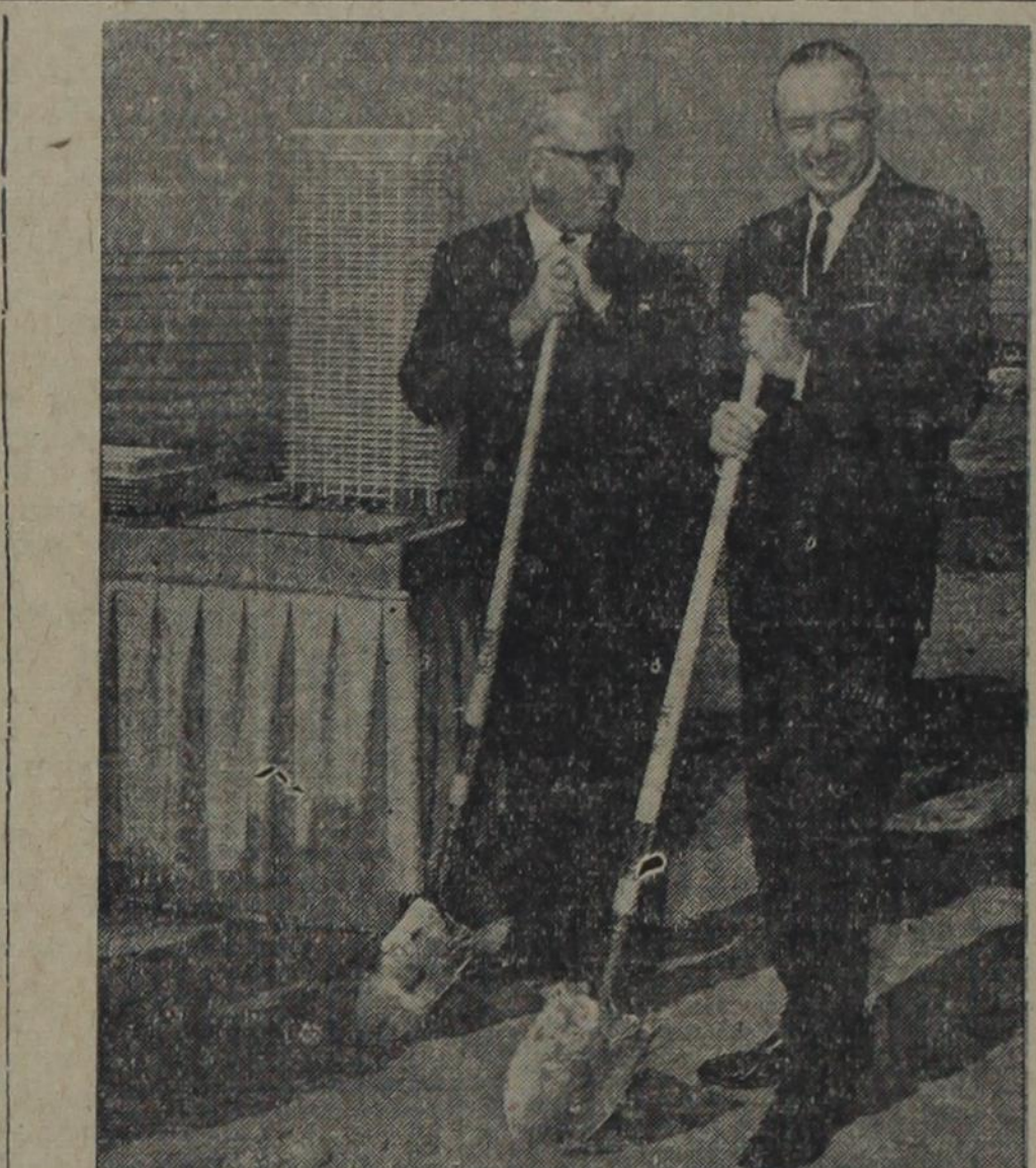
SPADEWORK ON HUMBLE'S NEW HOME—In Houston, Morgan J. Davis (right), president of Humble Oil & Refining Company, turns the first shovel of soil for Humble's new 4-story office building shown in the background model, while Humble Division President Ray E. Horton joins in the ceremony. The 600-foot structure, with some 1,000,000 square feet of usable space, is scheduled for completion in late 1962.
